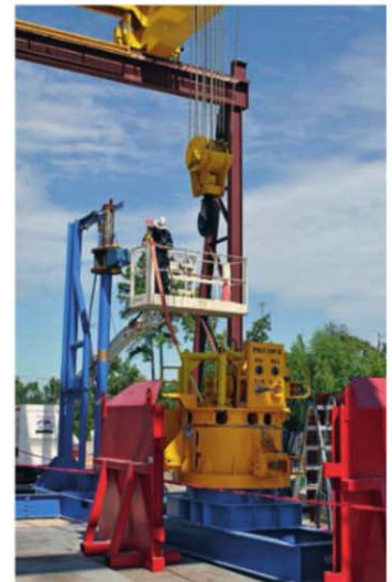
TEST TIME: The wellhead fatigue mitigation system is put through its paces in the system integration test to confirm operability and functionality.
